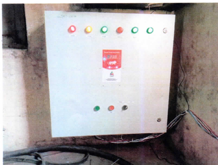
Scada Based Water Flow Control Panel
