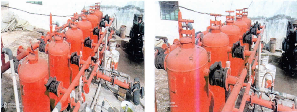
Filters and vanchury for centralized water Distribution
